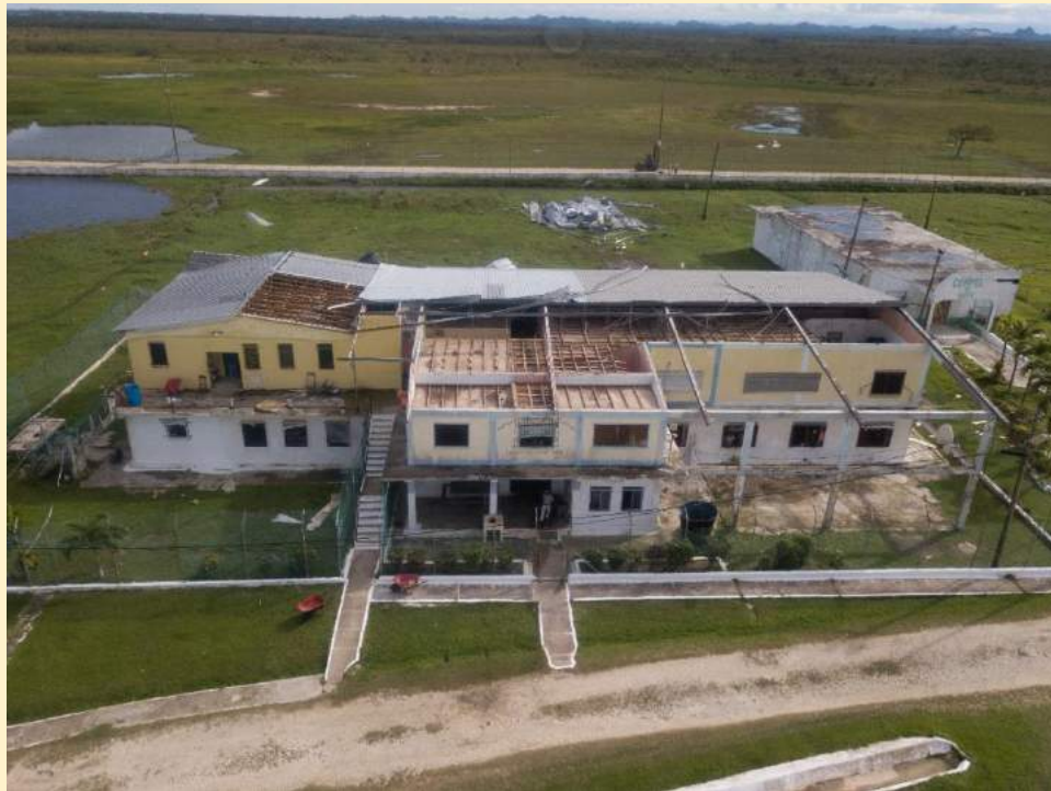
Rotary Learning Center roof torn off by Hurricane Lisa
