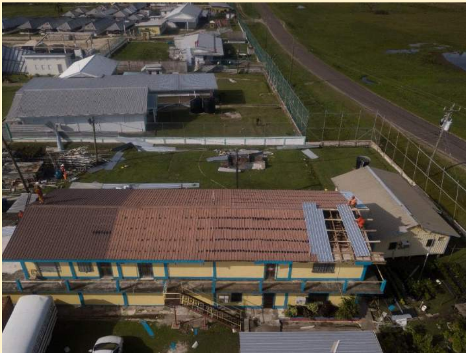
Roof damages to Records/Parole Offices
