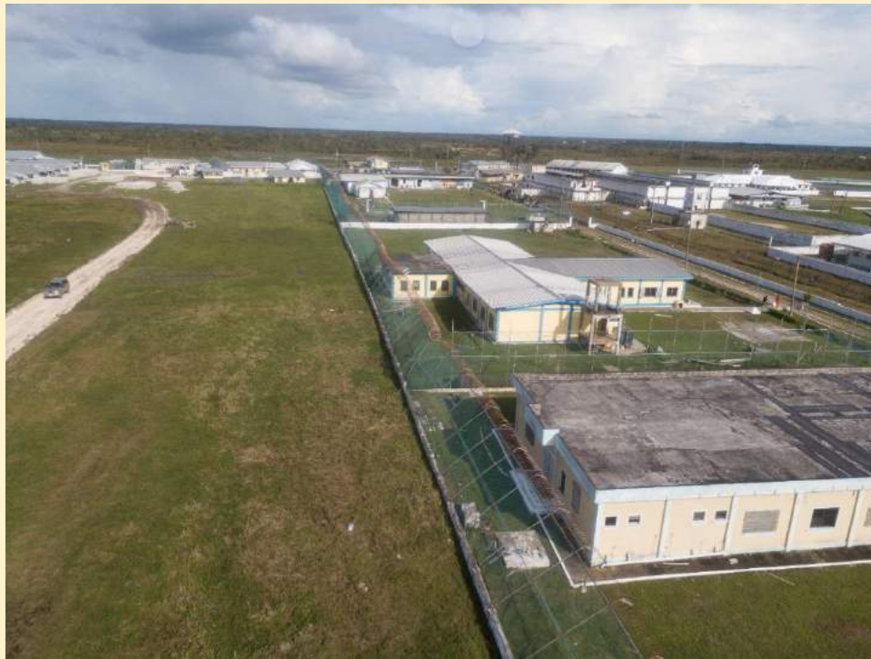
Outer Perimeter security fence behind ARC & CGS blown down by the hurricane
