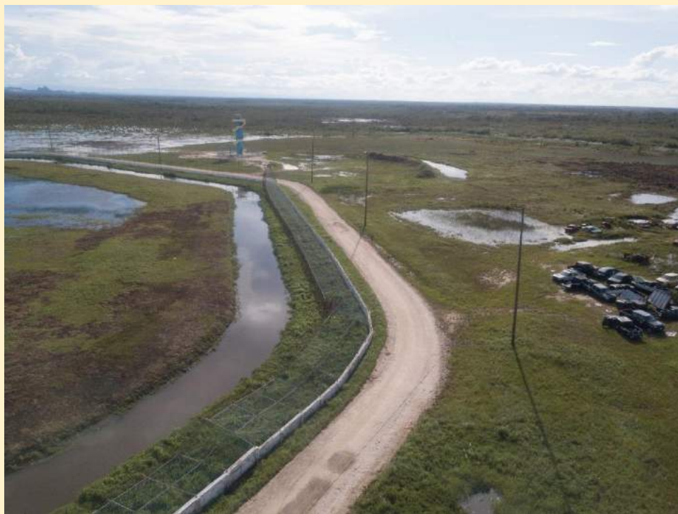
Outer Perimeter security fence behind the prison flattened
